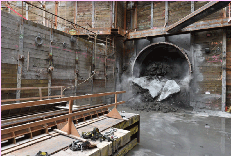
First Signs of the Break Through at the Same Location as previous photo!
