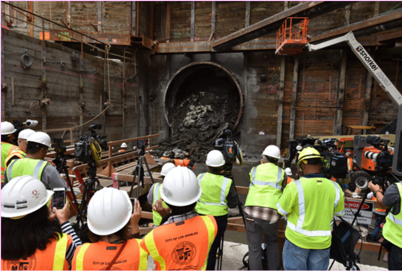
Crews Waiting with Anticipation for the Break Through at Second & Hope Streets. This will be the site of the Grand Avenue Arts/Bunker Hill Station.
